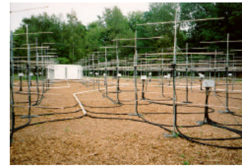
View through the antenna array at the radar lab
